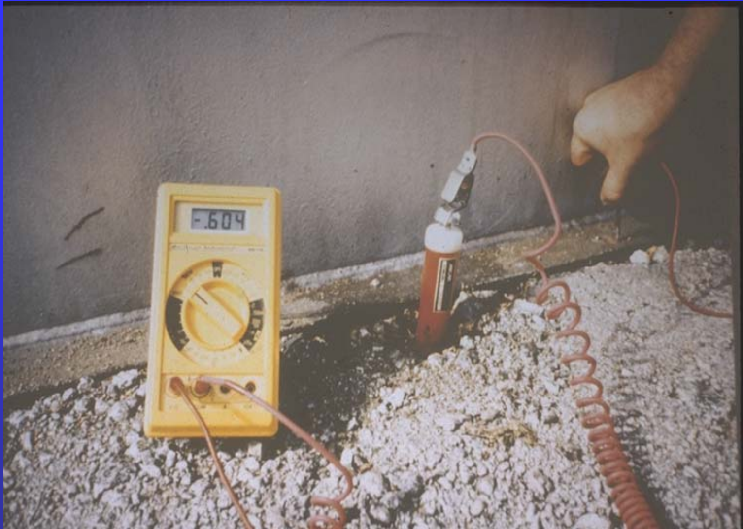
Tank to Soil Potential Measurements
