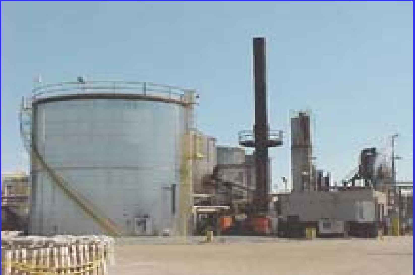
Hot Asphalt Tank Bottoms
